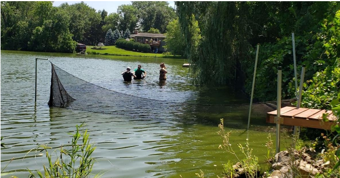
Figure 2: In the process of installation of the box net in the Northwest corner of Lake Nancy.
