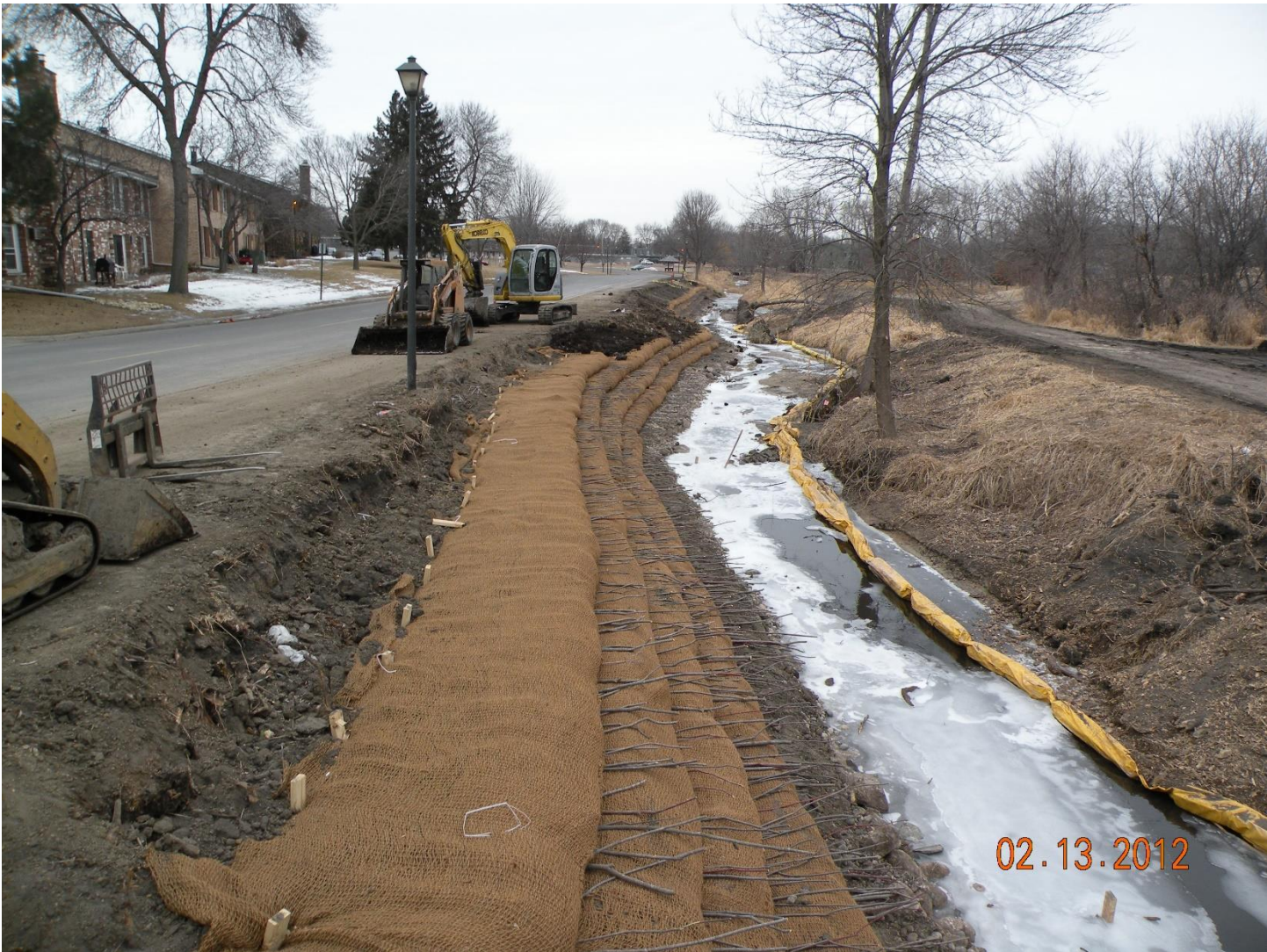
Work in progress in the City of Hopkins portion of the project
