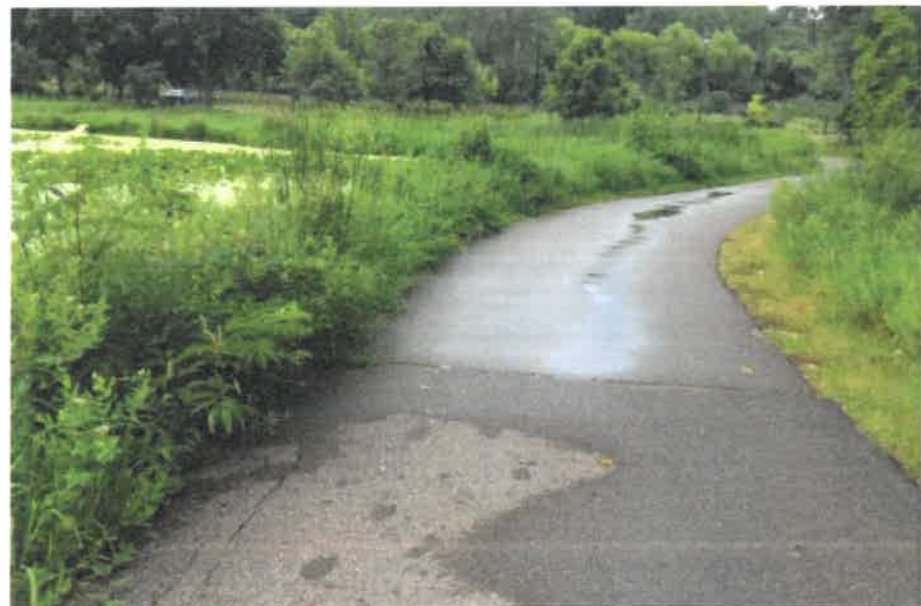
Existing trail, Lake side of trail has settled, trail patch repair, Existing buffer to be maintained, July 2018
