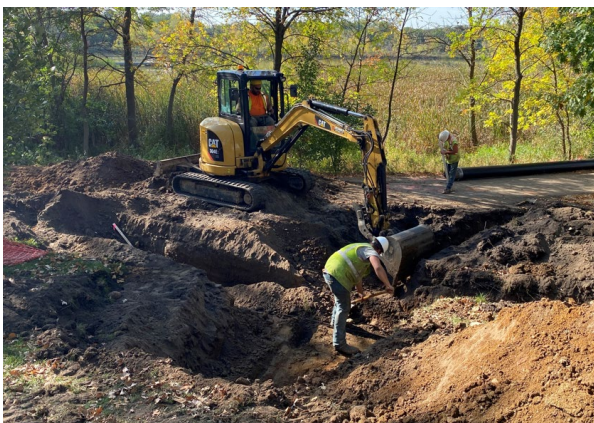
New outlet pipe to North Cornelia installed for treated water from the filtration vault
