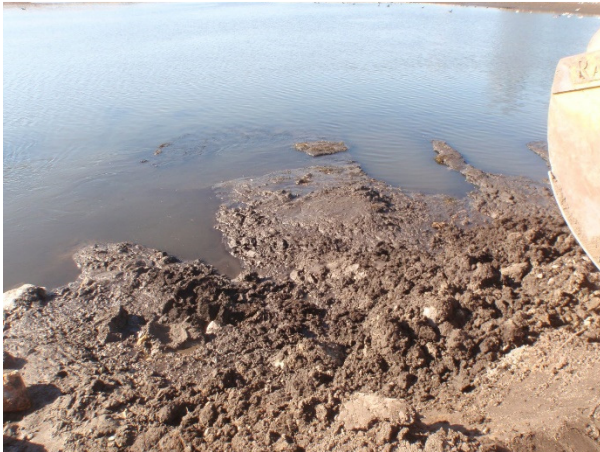
Soft sediments encountered at edge of construction access ramp extended into Normandale Lake.
