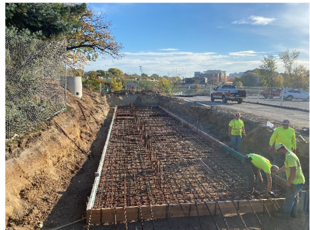
Installing rebar and preparing for pouring of the concrete in the filtration vault.
