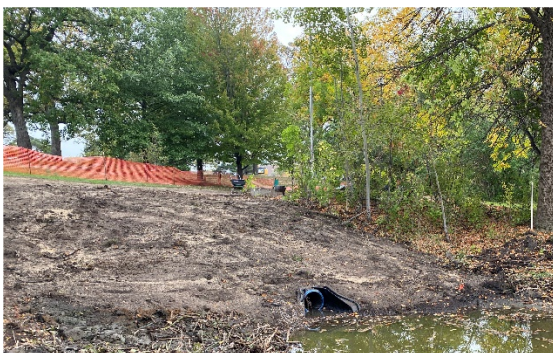
A new pipe is installed to convey filtered water from the treatment vault to Lake Cornelia.
