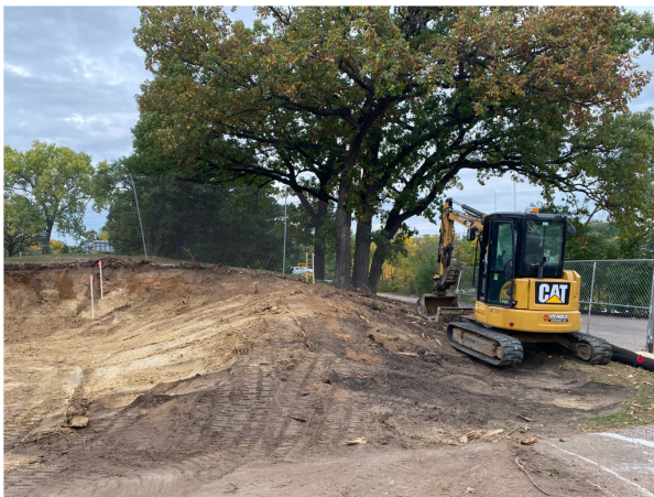
Pember starts construction of the Rosland Park BMP Project at the end of September 2021.
