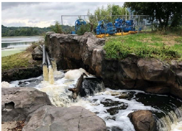
Pumps are discharging lake water downstream of outlet.
