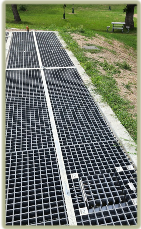
Figure 4-5 Pretreatment concrete vault with an open grate in Rosland Park (Edina)
