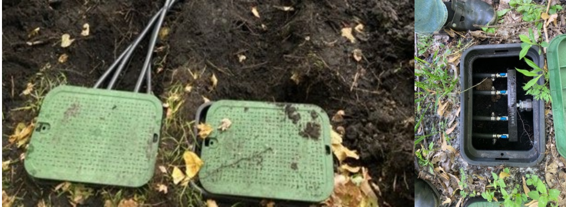
Figure 5-5 Example of a splitter box located downstream of the compressor and at the water's edge
