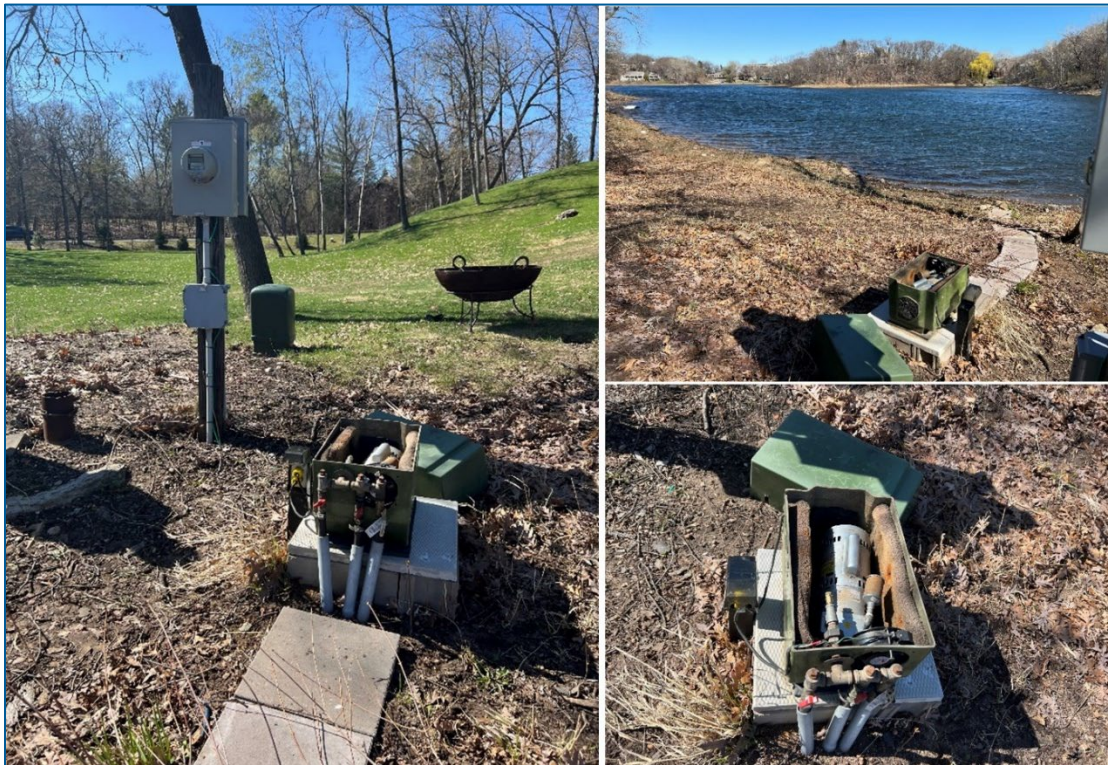
Figure 4-3 Existing Aeration System at Arrowhead Lake
