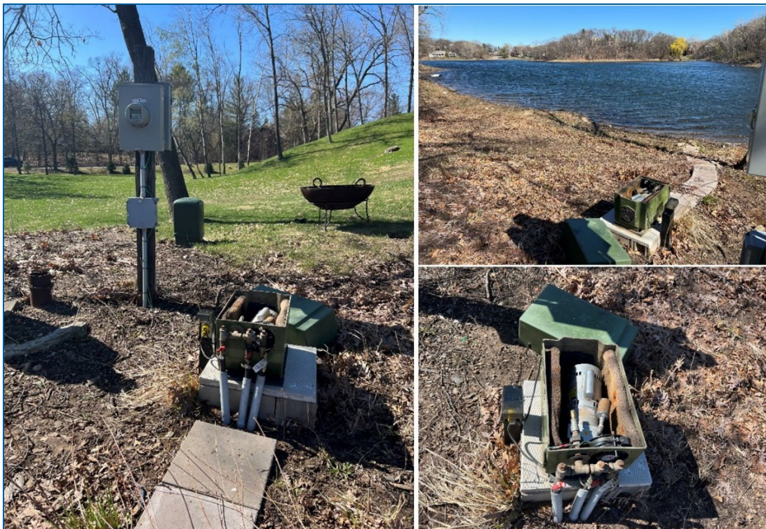
Figure 4-3 Existing aeration system at Arrowhead Lake
