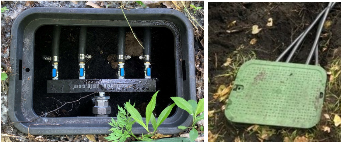
Figure 4-7 Splitter box and valves that control airflow to the aeration heads
