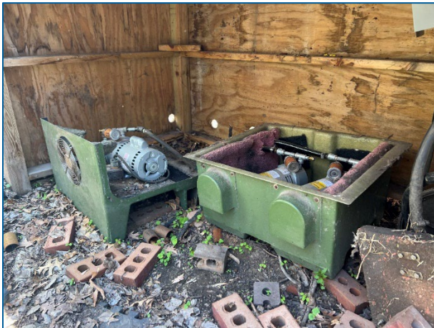
Figure 5-3 Existing compressors and housing system for the Indianhead Lake aeration system
