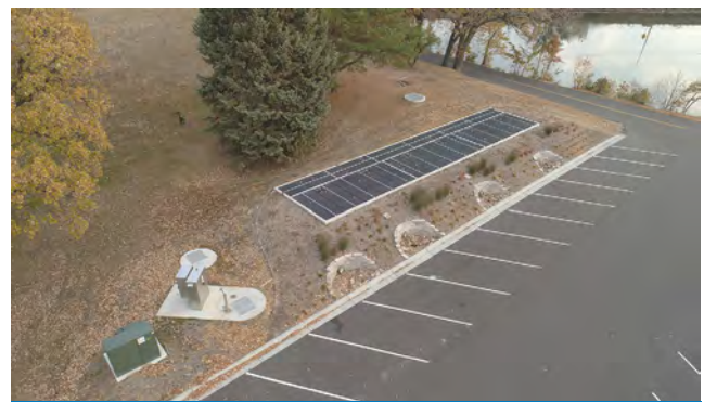
Rosland Park Stormwater Filtration Vault
