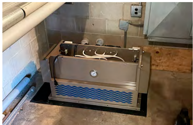
Aeration System installed on Lake Holiday
