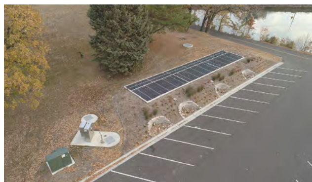
Rosland Park Stormwater Filtration Vault
