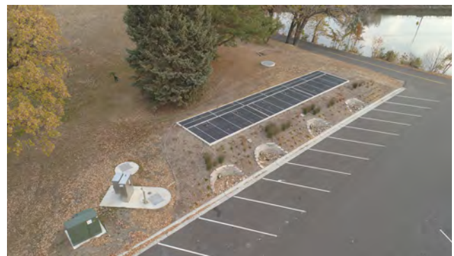
Rosland Park Stormwater Filtration Vault
