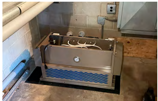
Aeration System installed on Lake Holiday
