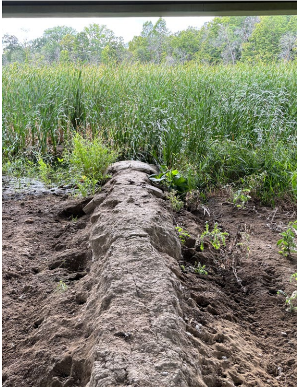
Figure 8-10 Settling and/or soil erosion around Southeast Anderson culvert (September 2025)
