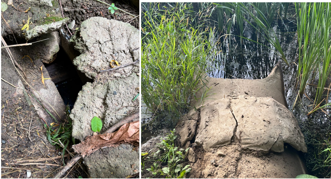
Figure 8-9 Degrading Southeast Anderson storm sewer infrastructure (September 2025)
